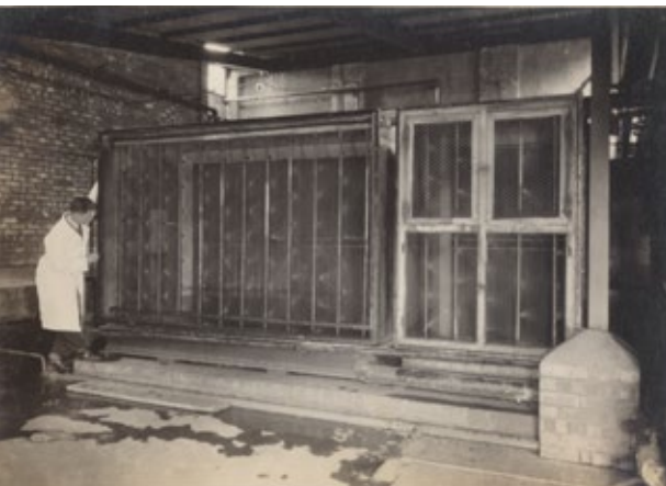
fig. 6 The Air-Washers at an Ilford Limited Factory, 1938. Photograph album of Selo Works in Brentwood (box1354), courtesy of Redbridge Museum and Heritage Centre (90/359/D2/A7).
