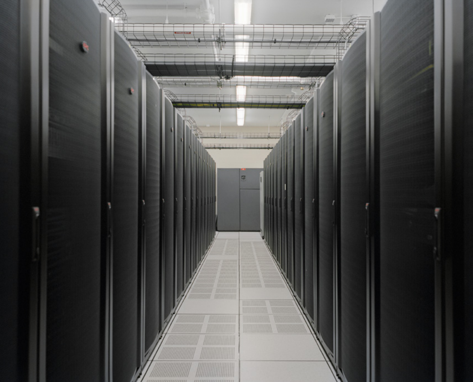
fig.4 Mark Kasumovic, Server Room ( Research University ), Western University, London, 2015.
