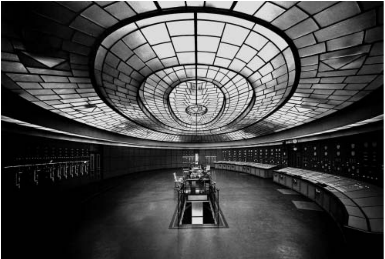
Tivadar Kozelka, Control room of the Kelenföld Power Station, Budapest 1933. Credit The National Office of Cultural Heritage
